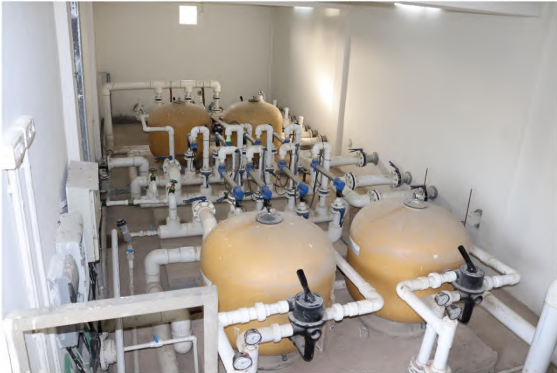
Figure 2.15: Water treatment facilities at Aquatic Reptile Rescue Facility of GZRRC
