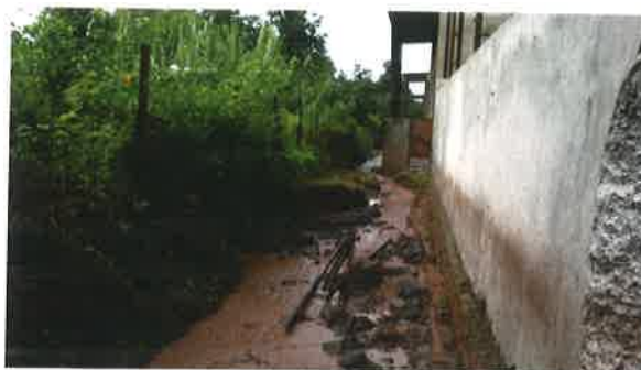
Damage to the Colony Aviary caused by floods
