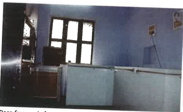
Deep freezers in freezer room
