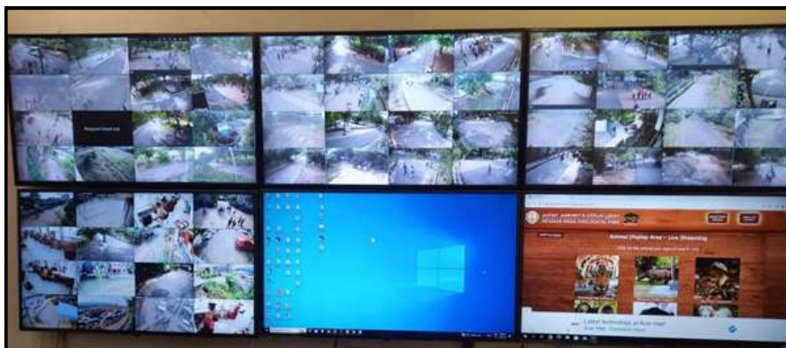
FIG. 45: CCTV CAMERA CONTROL ROOM
