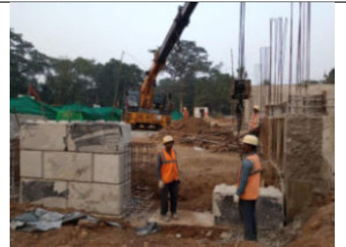
Under construction Lion exhibit at new site as per approved masterplan layout
