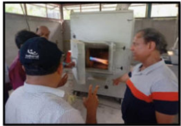
LPG based incinerator
