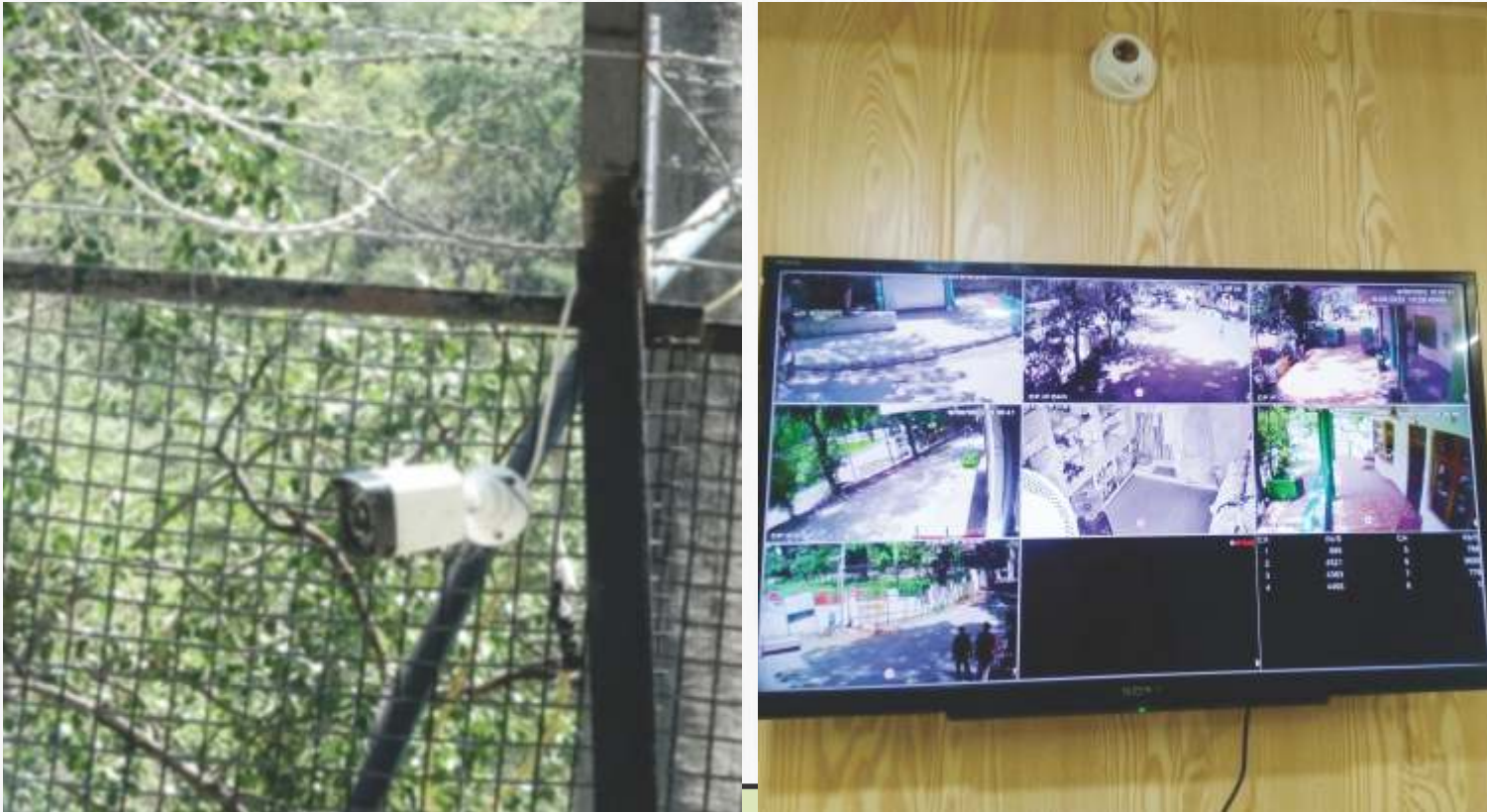
CCTV cameras installed along zoo enclosures
