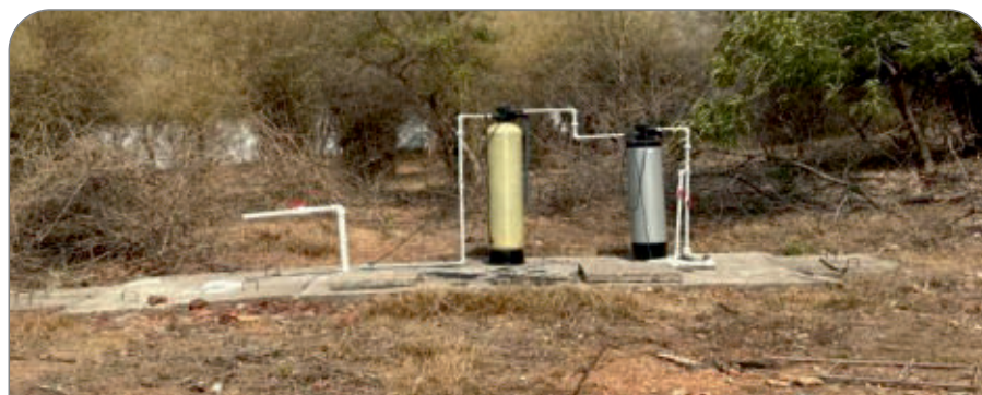
Waste Water Treatment Unit
