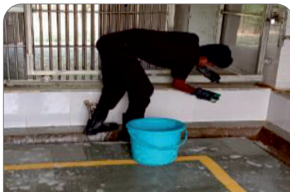
Cell Outside Cleaning
