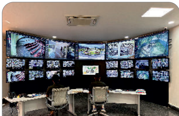
Control Room CCTV Monitoring Displays
