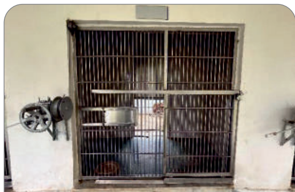
Drop gate operating system
