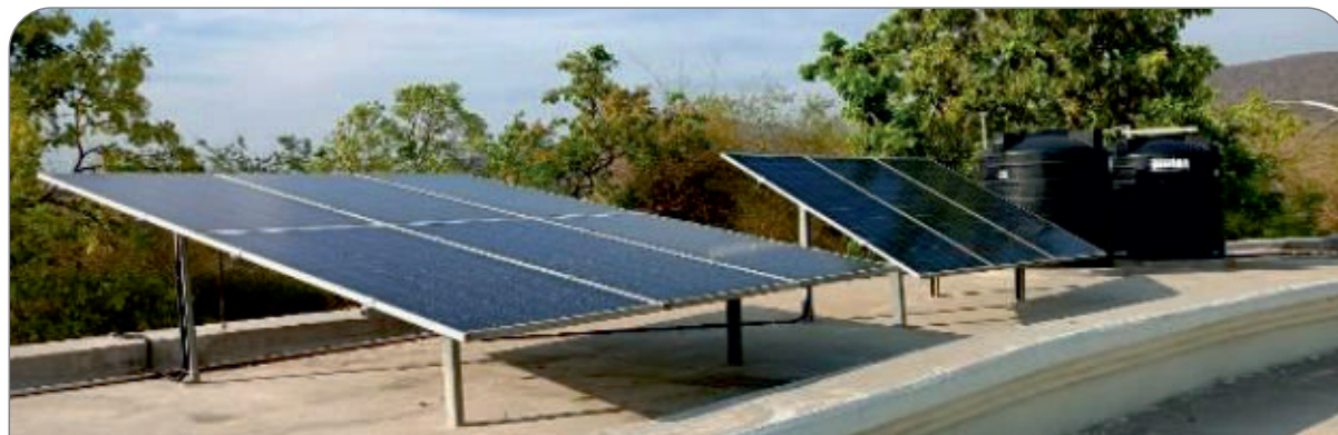
Solar and Water Tank
