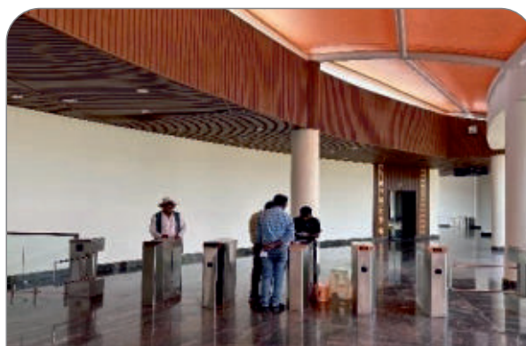
Ticket Checking Turnstiles
