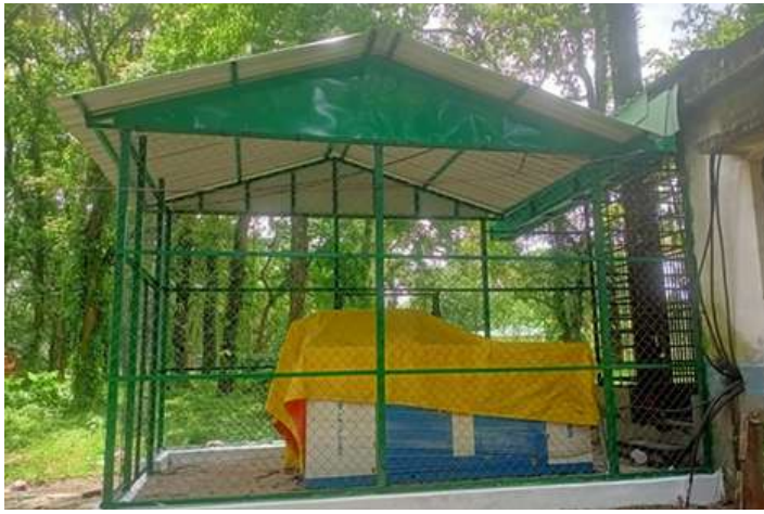
New generator house
