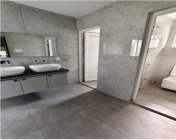
Renovation work for rest room of participants with toilet of admin block
