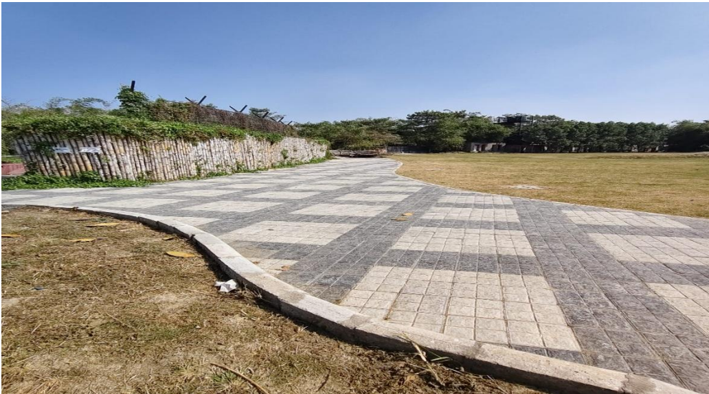
Extension work of brick works for service pathway from lion enclosure to emergency exit gate
