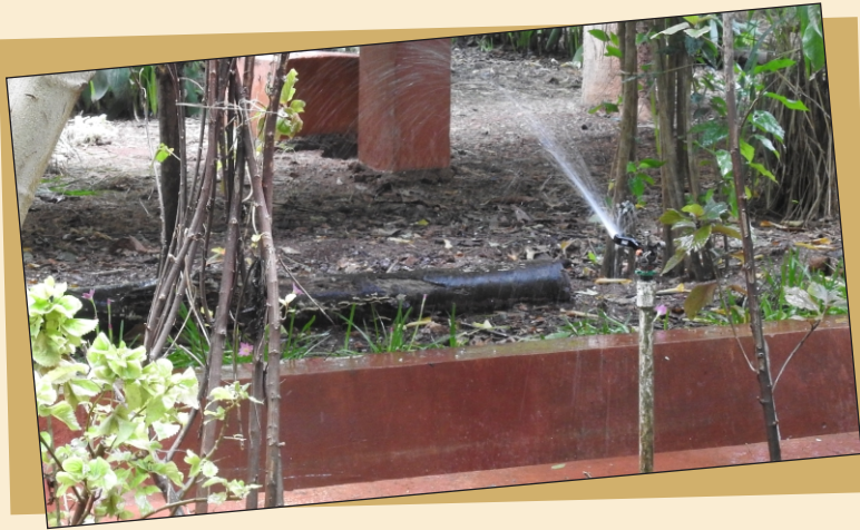
Sprinklers at various enclosures
