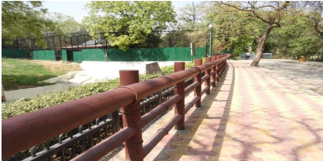
Replacement of damaged bamboo railing with M.S. Pipe railing of Royal Bengal Tiger Enclosure Beat No. 05
