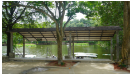
Boating shelter was restructured to provide a suitable waiting area for visitors during weather extremities.
