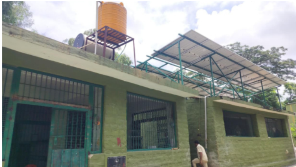
The existing safari day kraals were strengthened and restructured to enable safe and efficient management of resident tigers housed in the Indira Gandhi Holding House, along with the provision of solar-powered borewells.
