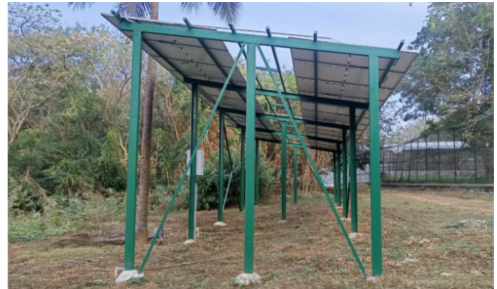
As an initiative to utilise ground water for the park maintenance, borewells were dug in the Host plant garden, Rescue Centre and Camp Office. Additionally solar power panels were installed to utilize renewable energy to pump the water.
