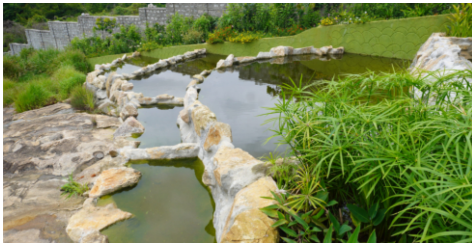
A filtration garden was set up near the boating area to facilitate rotation of the water by pumping it over a dedicated, multi level structures over natural rock with suitable aquatic flora to filter and aerate the water back into the boating area.
