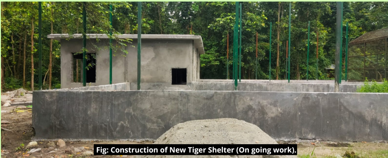
Fig: Construction of Security room at animal encloser & Twin quarter for Mahut and Patawala at Pilkhana.
