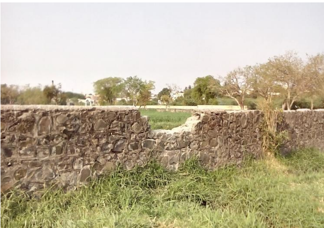
Figure: 1 - Old wall compound
