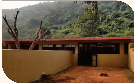
Construction of Night kraal to Sambar enclosure and renovation to Gaur night house
