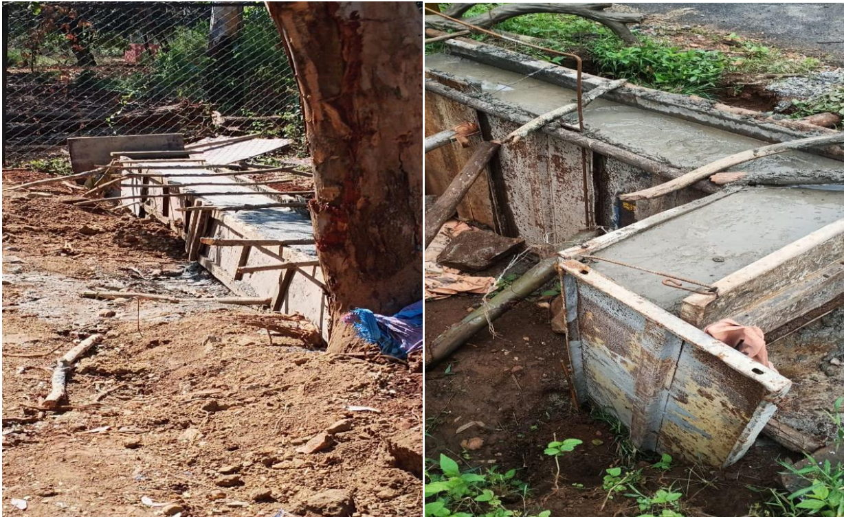
Construction of culvert at Tiger safari premises at Tiger and Lion safari Tyavarekoppa, Shimoga, during 2019-2020
