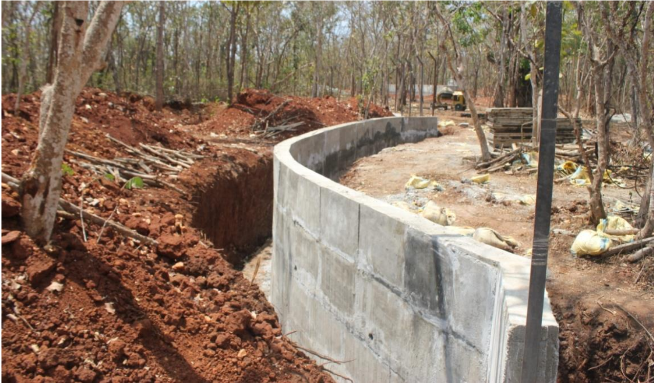
Construction of Ostrich enclosure and holding room, day kraal, moat wall, fencing, water supply work in Tiger & Lion Safari, during 2019-2020
