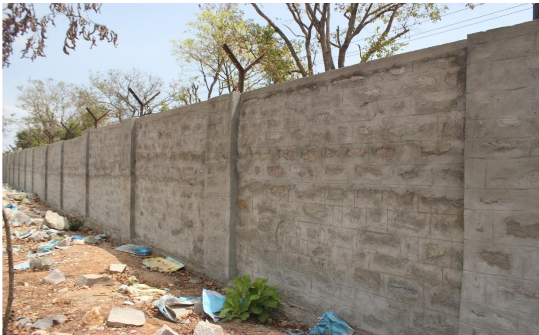
Construction of size stone masonry wall around safari enclosure adjoin to cultivated lands at private .Tiger and Lion Safari, Tyavarekoppa, Shimoga During 2019-20
