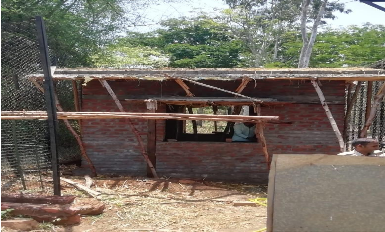
Construction of retaining wall near outer boundary at a chainage 2185.15 to 2242.20 in at Tiger & Loin safari, during 2019-2020
