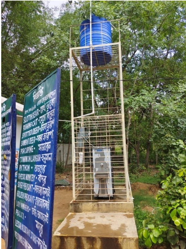
Drinking water at main entry gate for visitors
