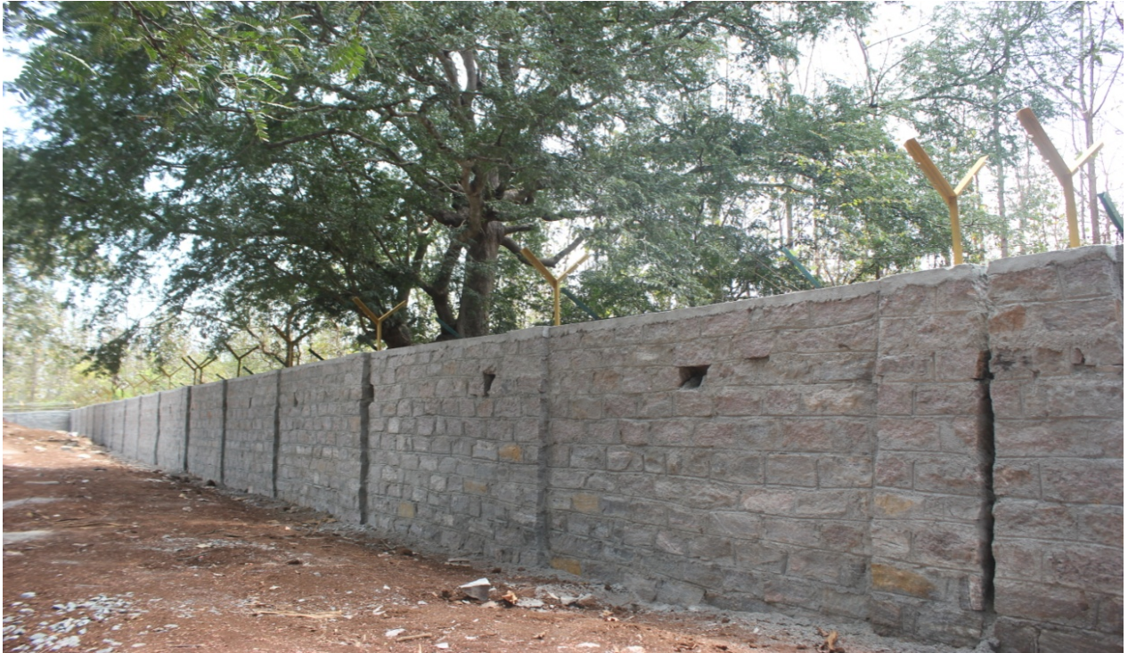
Construction of size stone masonry wall around Outer Boundary of Tiger & Lion Safari
