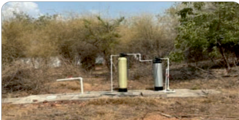
Waste Water Treatment Unit
