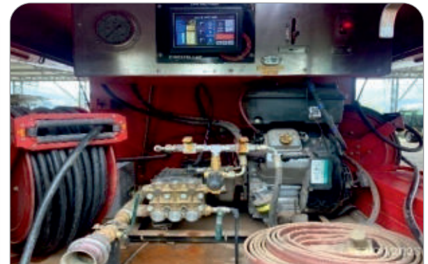
Fire Vehicle Interior
