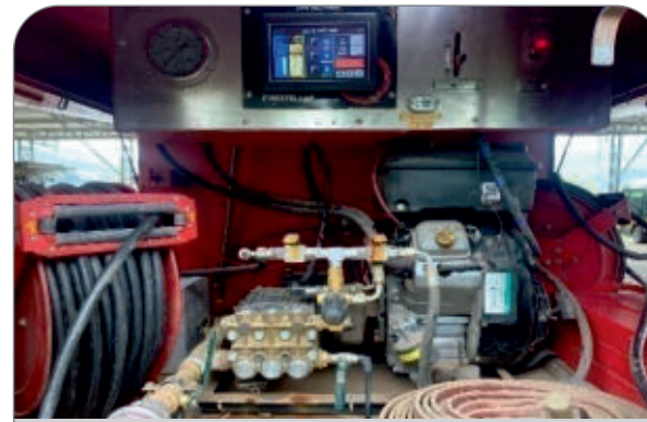
Fire Vehicle Interior
