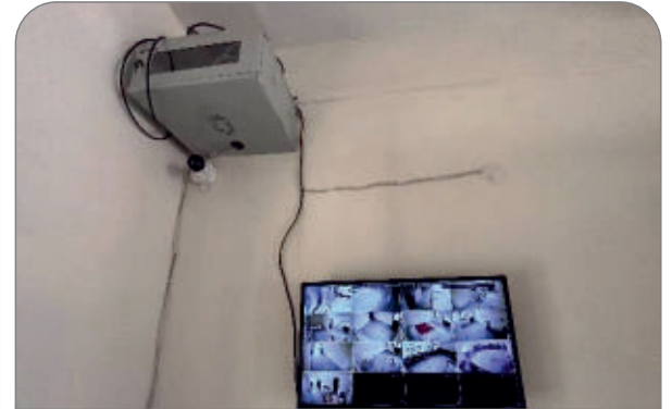
CCTV Camera with LED Tv
