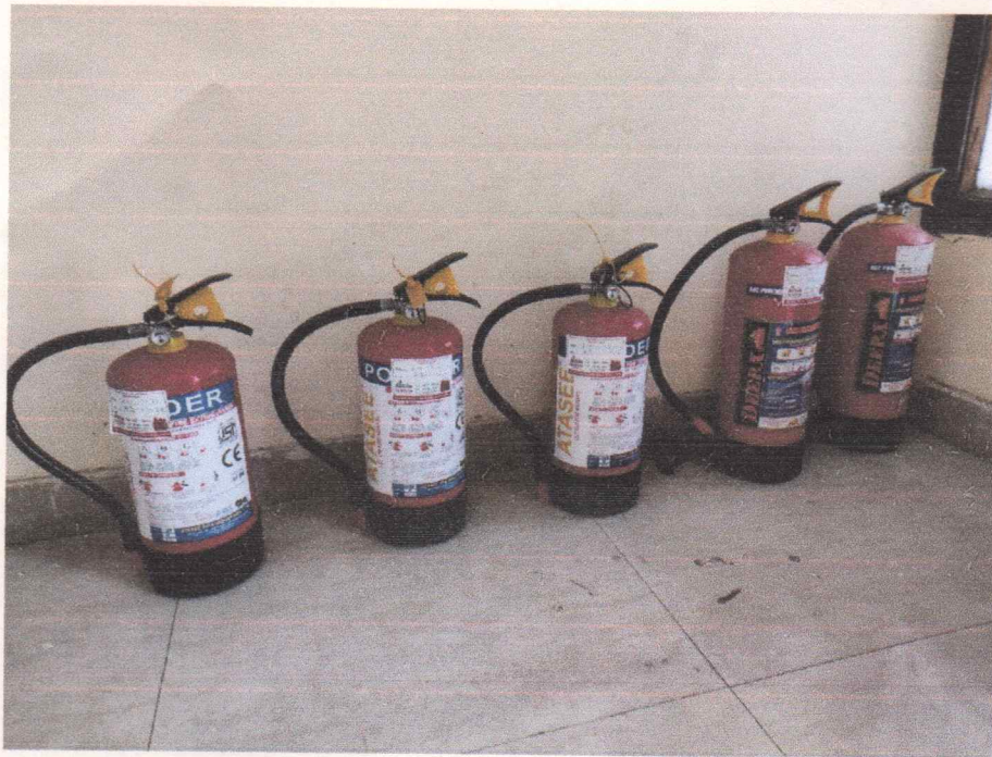
Fire Safety Equipments
