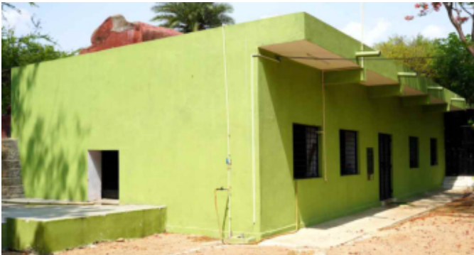
The old Sloth bear night houses were demolished and reconstructed with increased space for animal movement and an expanded keeper gallery to enhance safety and management efficiency
