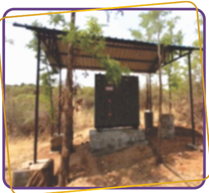
New Electrical panel
