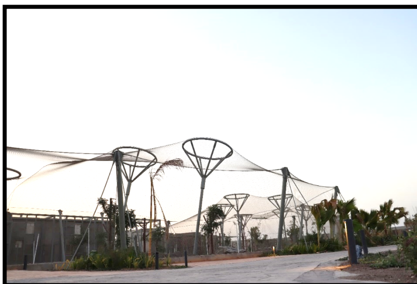
Woven wire mesh enclosure for Primates at Rescue and Rehabilitation Centre
