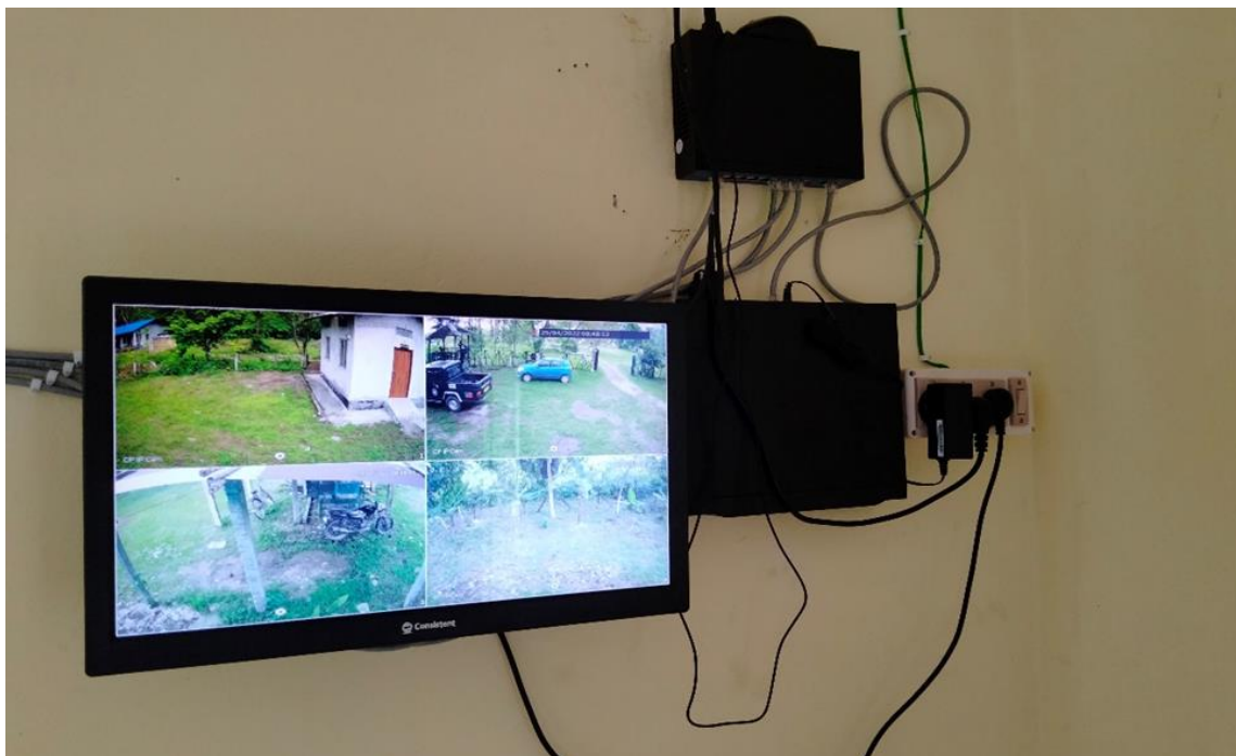
Figure 7: The operational hours of the office at the field station, which features a CCTV camera, are 24/7
