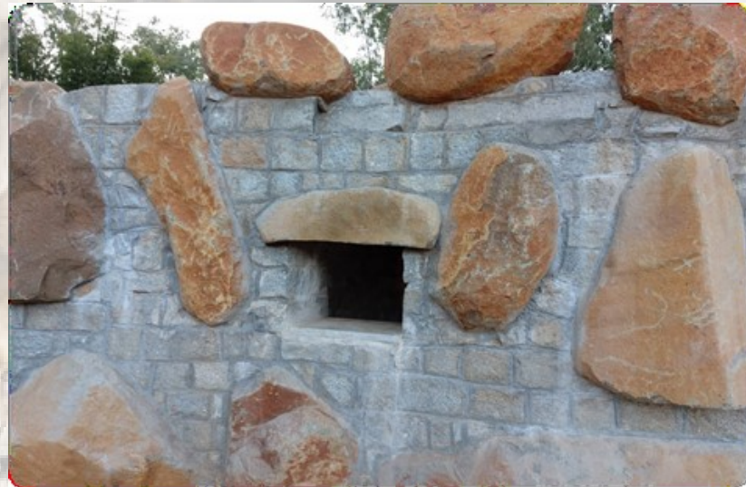
Constructing holding rooms and MOAT for BLACK BUCKS and LEOPARD HOLDING ROOMS
