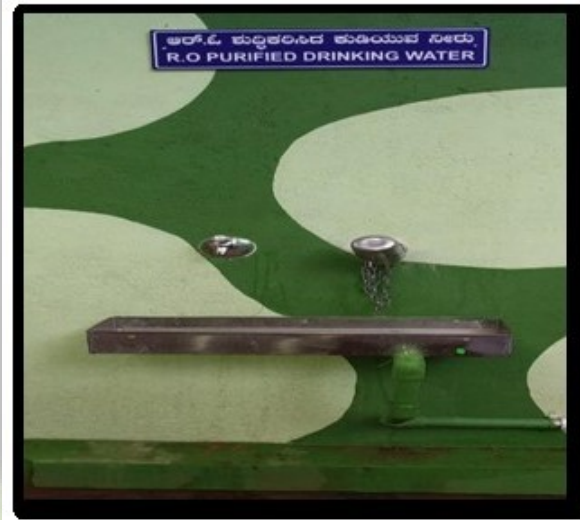
Sl. No: 37 - Drinking Water facility.
