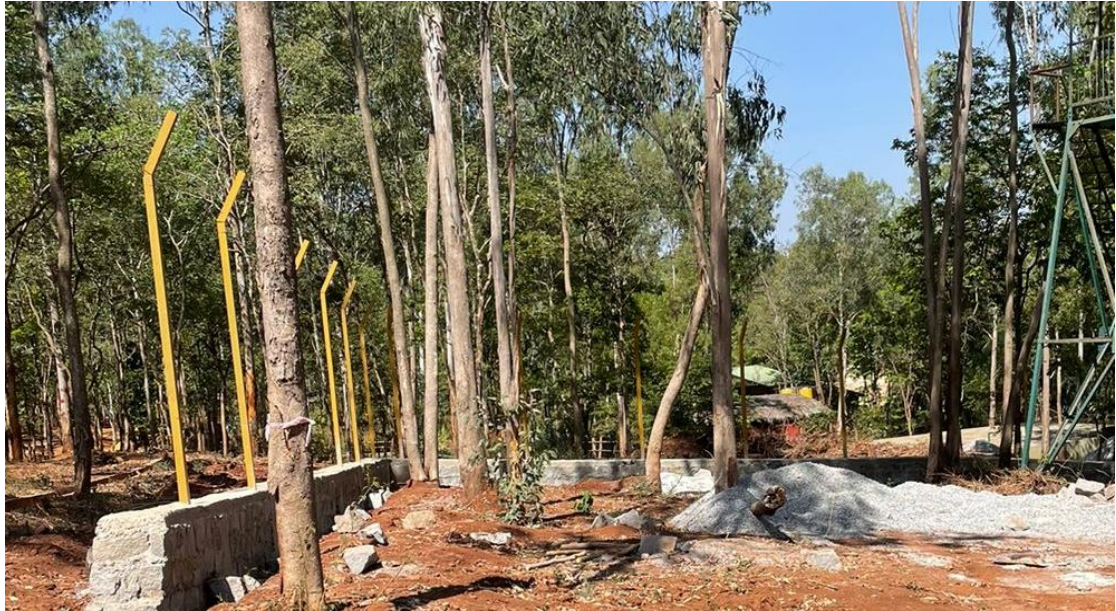
Construction of Zebra enclosure and holding house at Tiger and Lion safari, Tyavarekopa during 2022-23
