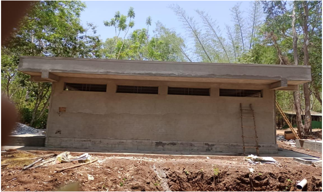
Construction of Toilet Block near exit at Tiger and Lion safari, Tyavarekopa during 2022-23
