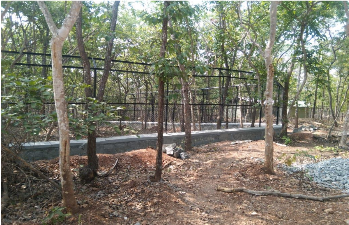
Construction of Blackbuck enclosure and holding house at Tiger and Lion safari, Tyavarekopa during 2022-23
