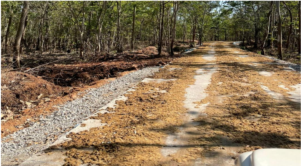
Construction of Road inside Gaur safari at Tiger and Lion safari, Tyavarekopa during 2022-23
