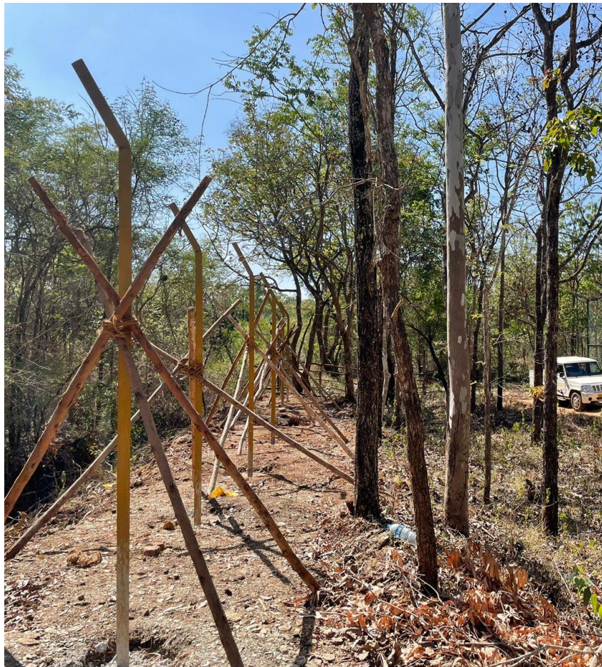
Providing Chain link Mesh along the outer boundary (Block 1V 1330.00 to 2920.00= 1590.00m) during 2022-23
