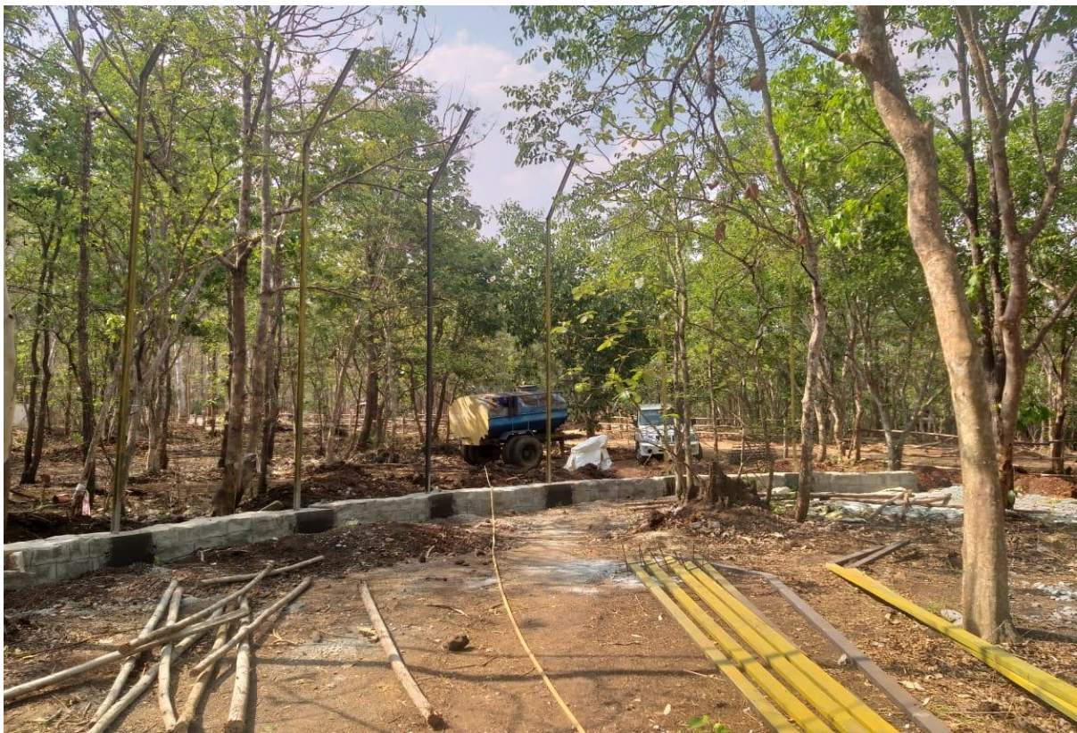
Construction of Assamese Macaque enclosure and holding house at Tiger and Lion safari, Tyavarekopa during 2022-23
