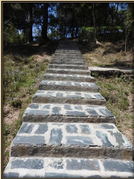
Picture 15: Replacement of stone tiles with traditional anti-skid stones keeping in view the safety of visitors.
