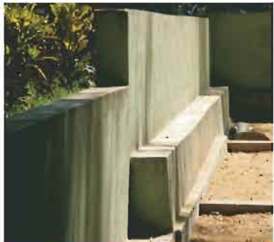
Steps in the enclosure wall can lead to an easy escape and should be avoided.
