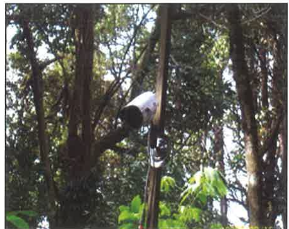
Fig. 26: CCTV Camera inside Enclosure
