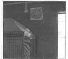
Fans for fresh air
