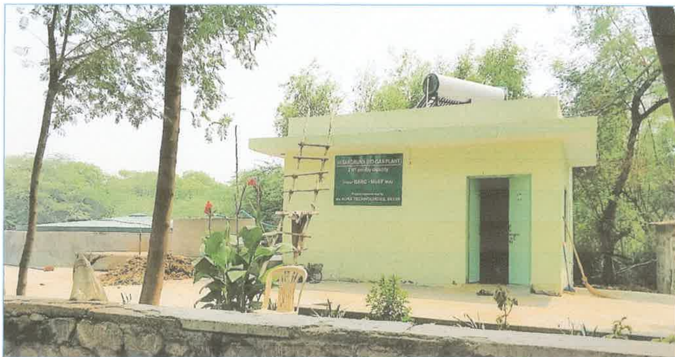
Bio-gas plant installed at NZP
